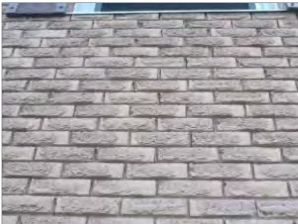
View of step cracking and differential movement noted in the brick masonry on the west elevation of block 15.
