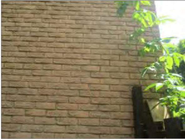
View of step cracking and differential movement noted in the brick masonry on the north elevation of block 5.
