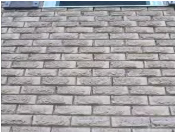
View of step cracking and differential movement noted in the brick masonry on the west elevation of block 15.
