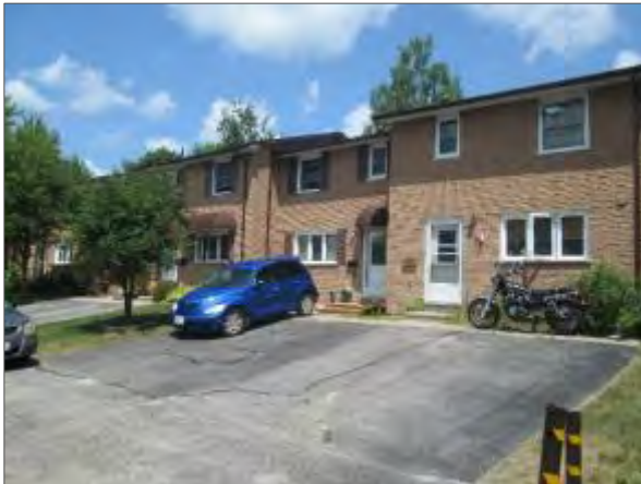
View of the typical asphalt paved driveways serving the units with typical pattern cracking observed.
