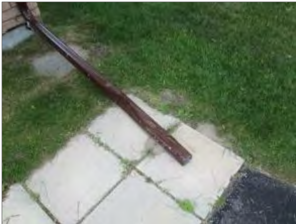
View of a typical crushed downspout extension.
