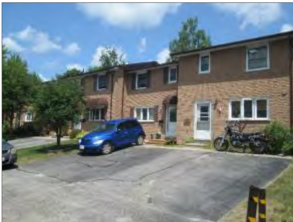
View of the typical asphalt paved driveways serving the units with typical pattern cracking observed.
