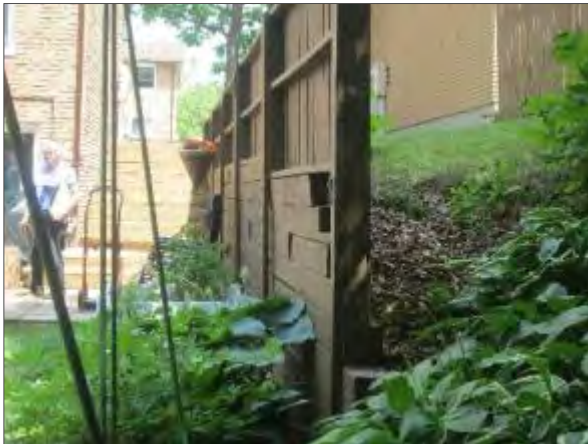
View of the wood framed retaining wall between blocks 7 and 8 which was noted to be leaning and will require replacement in the short term.
