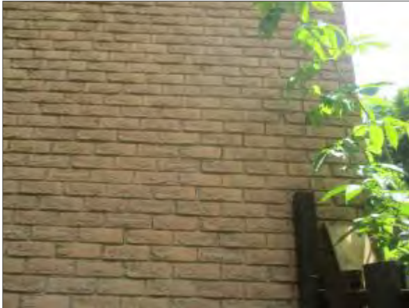
View of step cracking and differential movement noted in the brick masonry on the north elevation of block 5.
